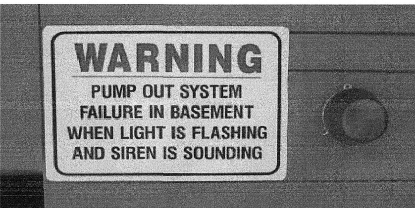
PUMP FAILURE WARNING SIGN AT BASEMENT ENTRY
